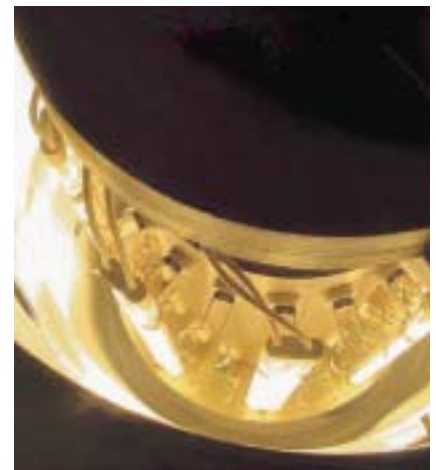
Interior heating of compressor housings
